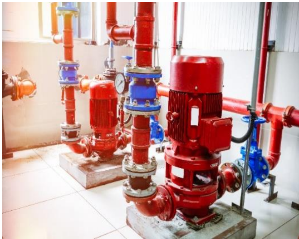
Fire Protection Booster Pumps
